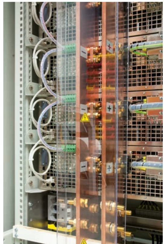
DC bus terminal
